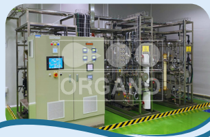
Project name: Water for injection Location: Thang Long IP, Hanoi Capacity: 1m3/h Year of completion: 2022
