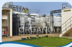
Project name: Wastewater treatment plant (CN & NI) Location: TLIP II, Hung Yen Capacity: 410m3/day Year of completion: 2012
