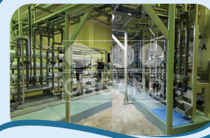
Project name: DI Water Treatment Plant for Thermal Power Plant Location: Phu My 1, Phu My Town, Tan Thanh Capacity: 6.5m3/h Year of completion: 2021
