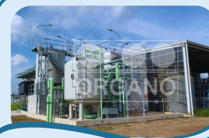
Project name: Wastewater treatment plant Location: TLIP II, Hung Yen Capacity: 80m3/h, 1760m3/day Year of completion: 2021
