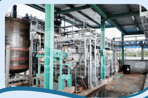
Project name: Wastewater treatment plant Location: Quang Minh IP, Me Linh Capacity: 261m3/day Year of completion: 2018
