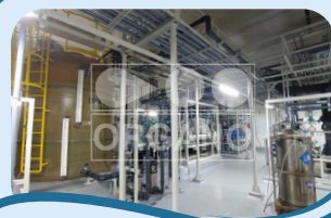
Project name: RO and Ultra Pure Water for Semi-conductor Location: Vietnam-Singapore IP Binh Duong Capacity: 15m3/h Year of completion: 2018
