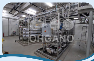
Project name: Water for injection Capacity: 4m3/h (phase 1), (expanded in phase 2) Year of completion: 2022
