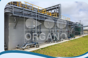
Project name: Wastewater treatment plant Location: Dinh Vu IP, Hai Phong Capacity: 135m3/day Year of completion: 2018
