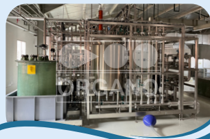
Project name: Purified Water System Location: JI. Pasteur Capacity: 5.0 m3/h Year of completion: 2022
